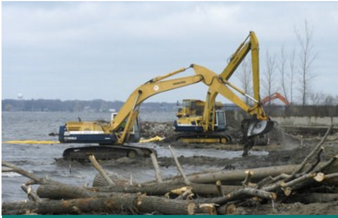
Construction taking place to restore degraded habitat at the Muskegon Lake Area of Concern.
