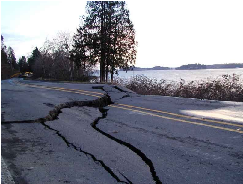
Figure SH.4. Image taken near Allyn, Washington, showing damage to the road following the 2001 Nisqually earthquake (6.8M). Impacts to remote coastal communities could be more significant, especially following a 9.0M earthquake, including critical failure of roads and bridges connecting these isolated communities. Photo: U.S. Geological Survey
