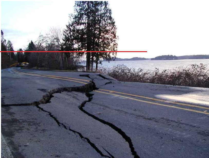
Figure SH.4. Image taken near Allyn, Washington, showing damage to the road following the 2001 Nisqually earthquake (6.8M). Impacts to remote coastal communities could be more significant, especially following a 9.0M earthquake, including critical failure of roads and bridges connecting these isolated communities. Photo: U.S. Geological Survey
